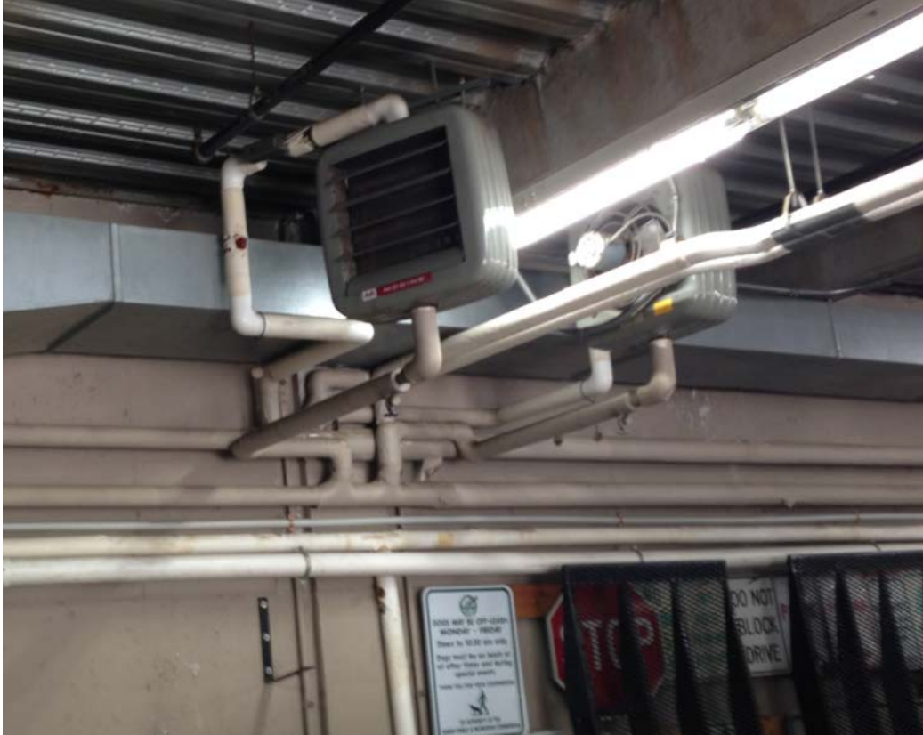
Typical Hot Water Unit Heaters
